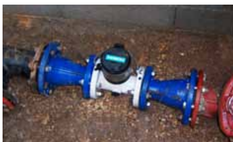
Bulk water / revenue metering: MAG 8000 monitors consumption accurately and economically
